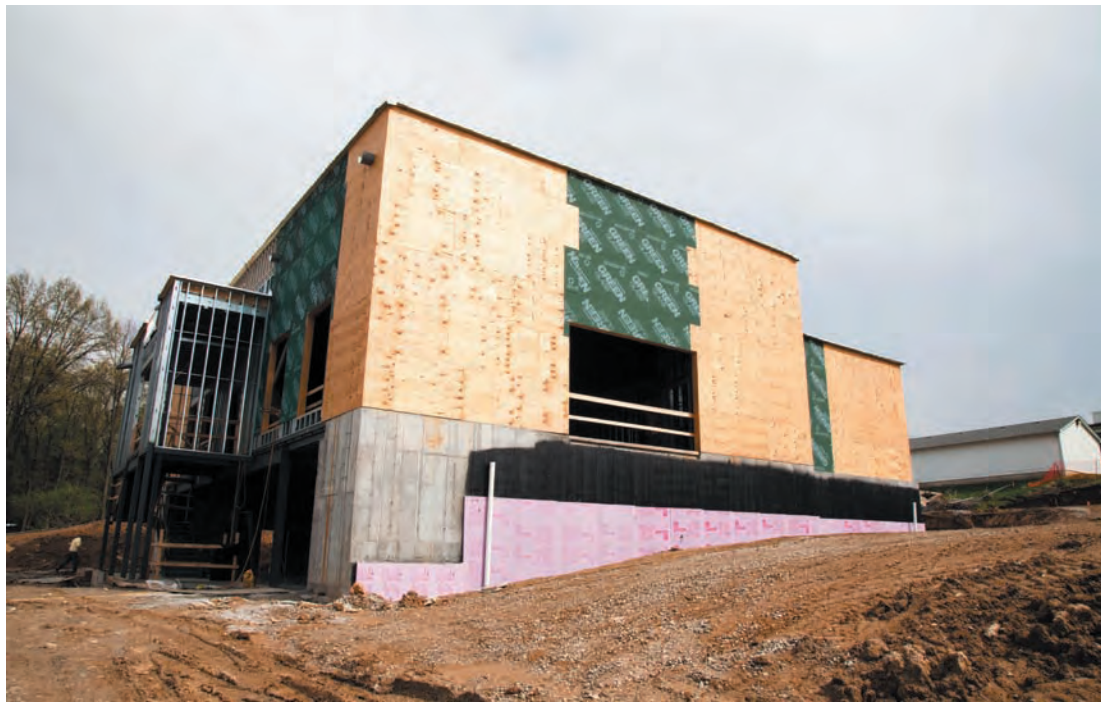
Nusach Hari B'nai Zion's new building, being constructed near Old Bonhomme and Price roads has incorporated green technology into its design. Photo: Kristi Foster.
